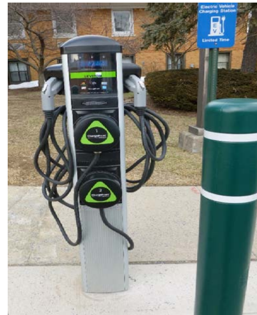
Level 2 Charging Station
