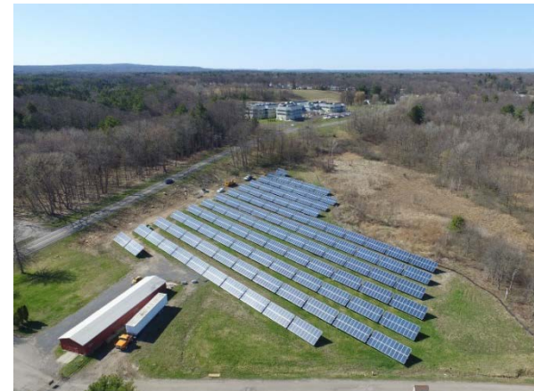
Schenectady County Recycling and Composting Center 600 kW
