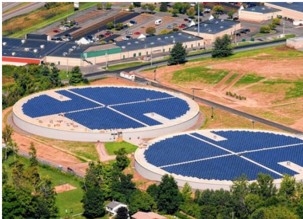
Onondaga County Metro Water Board Reservoir 2,000 kW
