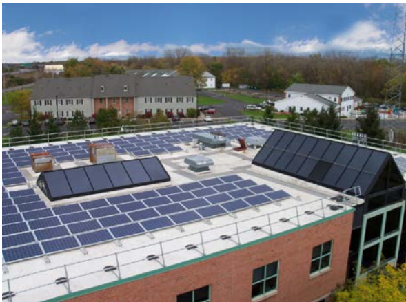
DeWitt Town Hall 50 kW
