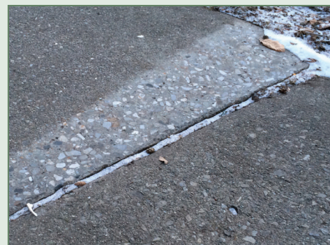
A sidewalk in the Village of Millbrook that has been shaved to even out the surface where lifting occurred.
